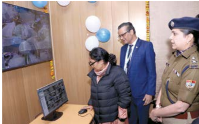
CCTV Surveillance System installed & commissioned by BEL in Kotdwara, Uttarakhand, was handed over to Kotdwara State Police in the presence of Hon'ble Speaker, Uttarakhand Legislative Assembly
